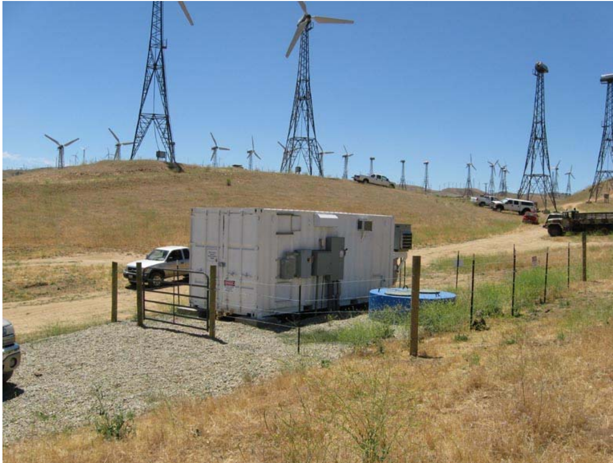
Tehachapi Installation – Control Enclosure w/ Flywheel Unit in Ground
