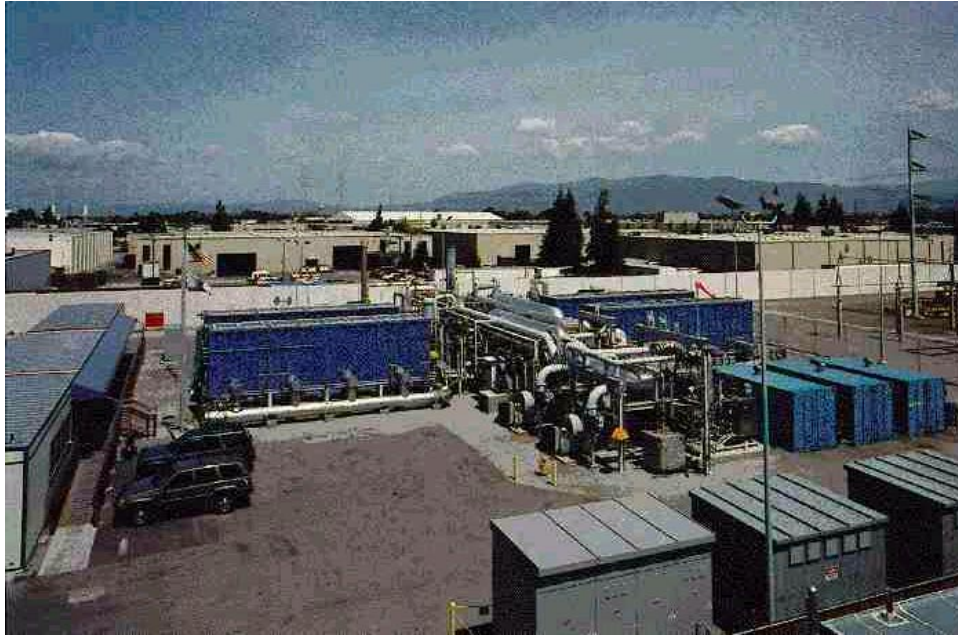
Figure 13 - Santa Clara MCFC Power Plant
