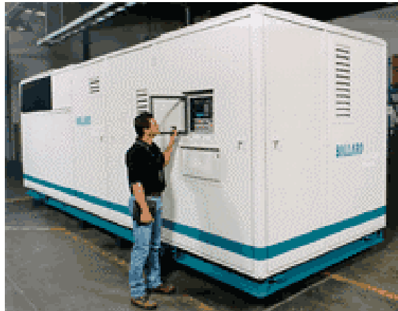
Figure 9 - Ballard Generating System's 250 kW PEMFC Unit
