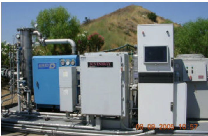
Figure 5. Gas Treatment Skid
