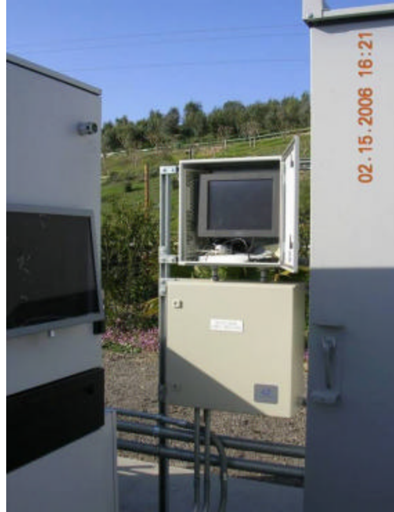
Figure 9. Smart*DER Computer Installation
