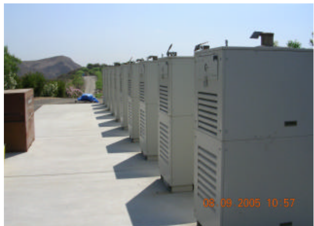
Figure 1. Calabasas Landfill - Microturbine Enclosures
