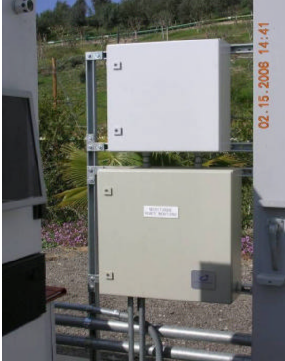
Figure 8. Smart*DER and Connected Energy Installation
